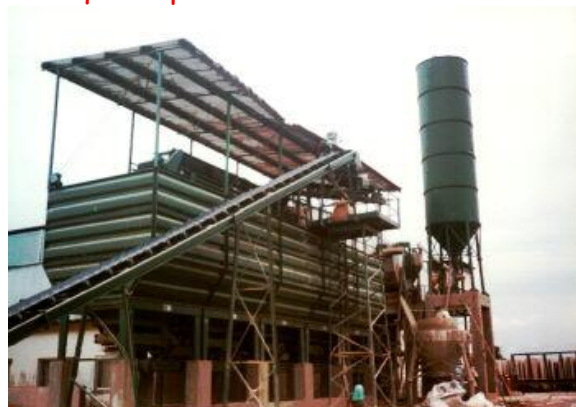
Concrete Batch Plant 50 cm/hour
